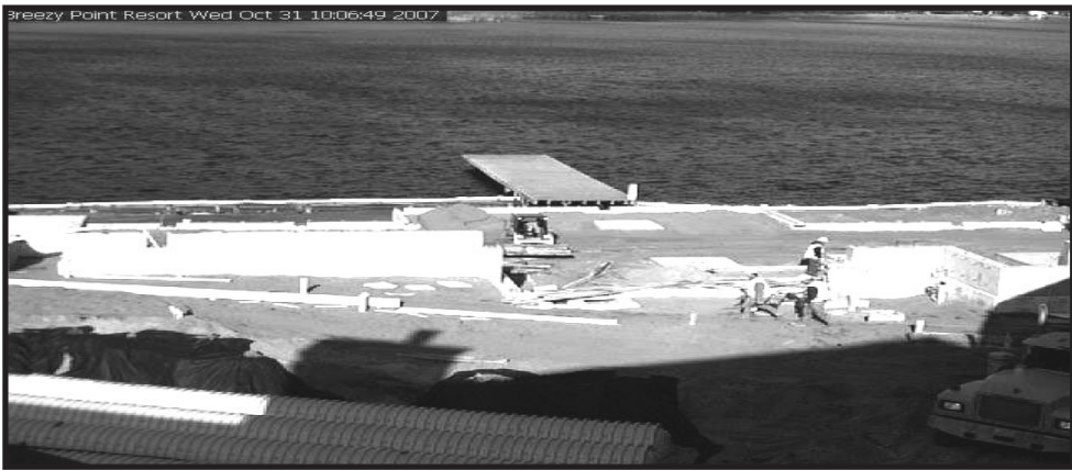
This is an October 2007 webcam picture of the site preparation for the new restaurant. The large pipes in the lower left formed a part of the storm water runoff system.
