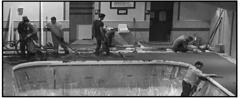
Workmen replace decking around the swimming pool and resurface the pool in the Recreation Center.
